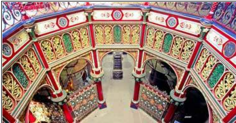
Crossness Pumping Station designed by Joseph Bazalgette.
